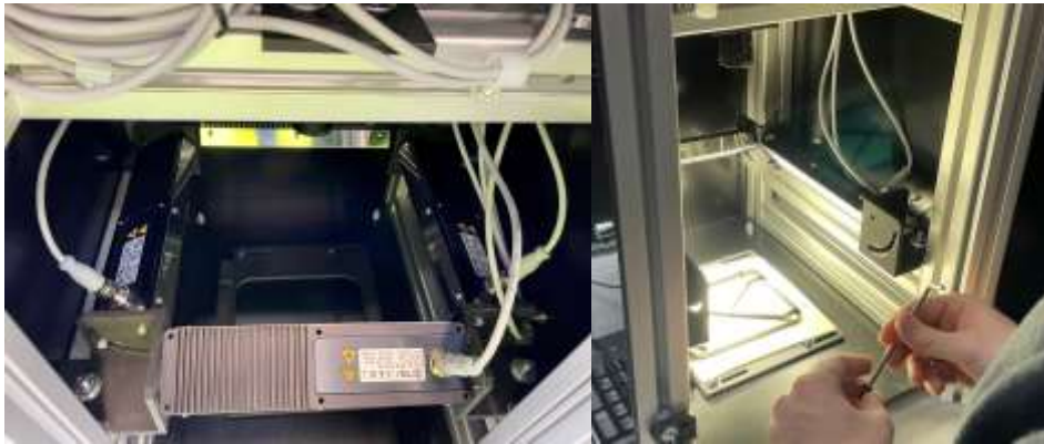
Figure 1: (Left) Illumination configuration; (Right) System getting installed by AIMEN
